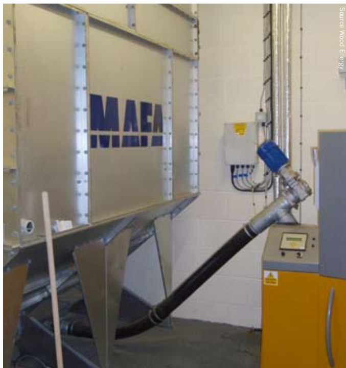
Galvanised and tapered pellet fuel store and boiler
