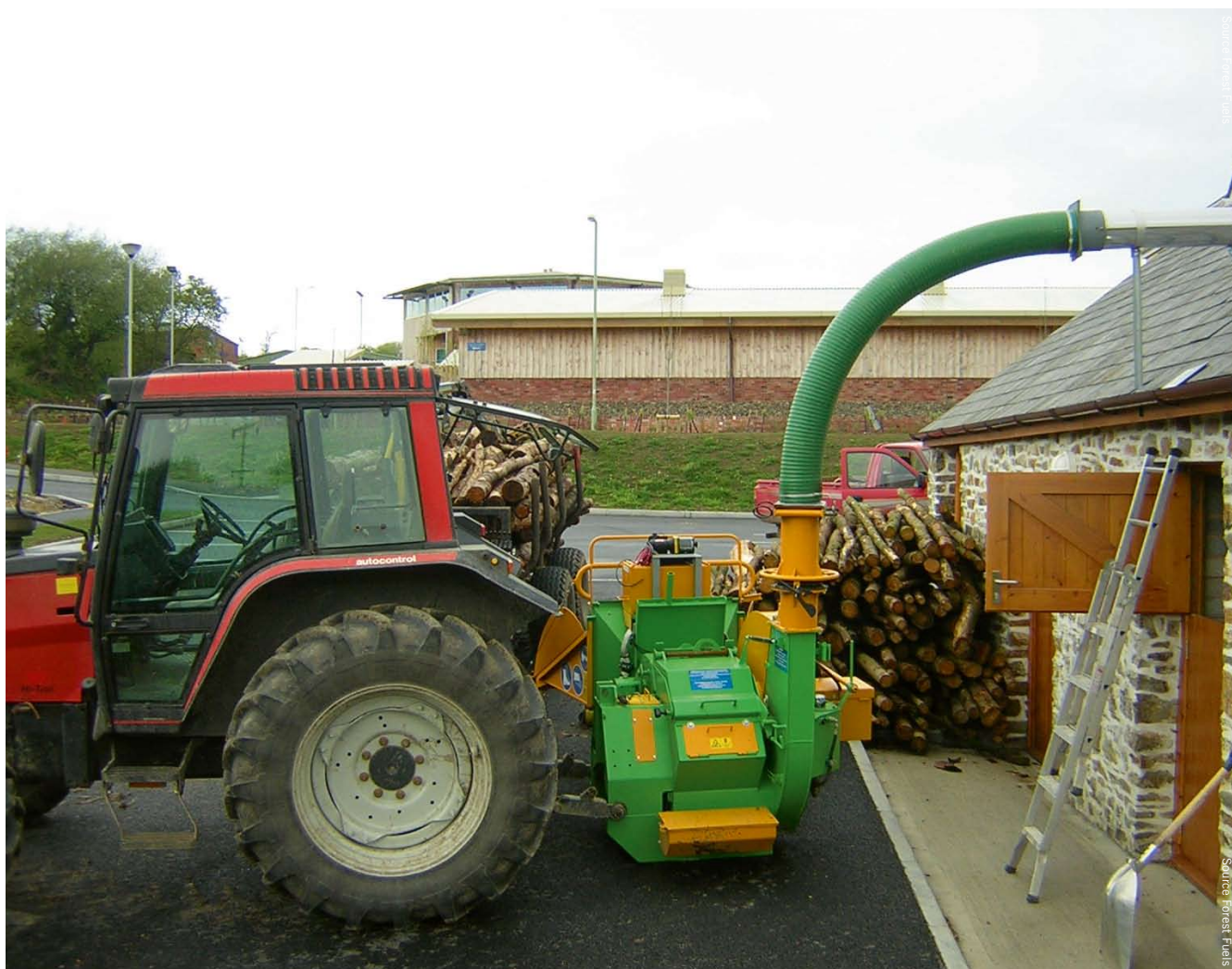
Direct chipping into fuel store – useful option where noise of chipping and timber storage is acceptable or as in this case where no other option is available due to limited delivery access via pedestrian door.
