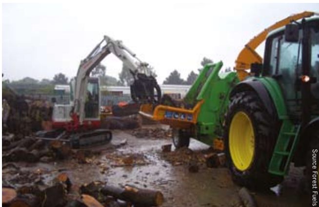
Excavator feeding chipper with arboricultural arisings of all shapes and sizes which would be difficult to crane feed with a conventional timber grab. Oxford City Council Tree Station
